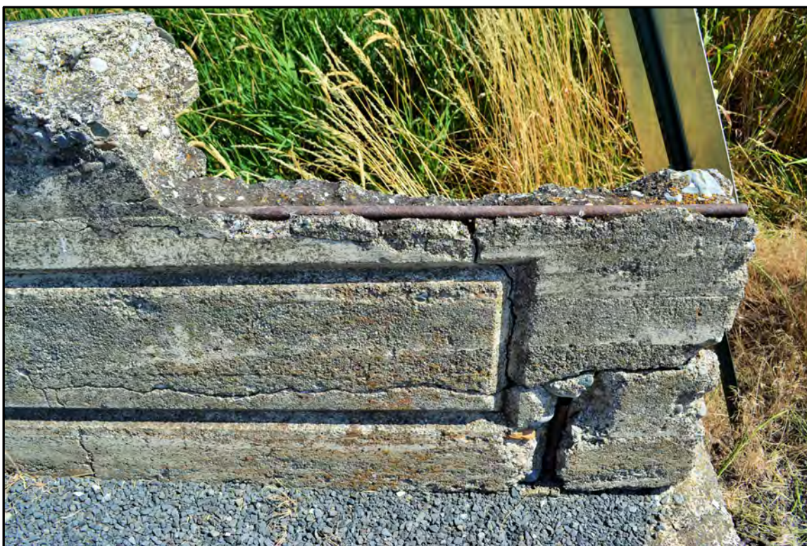
Figure A-40. Colton Bridge (Field Number WCLB-6), reinforcing rod exposed at south end of east balustrade; view to the southeast.
