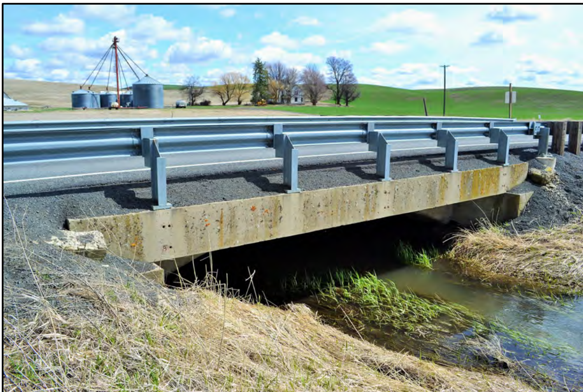
Figure A-24. Morley Bridge (Field Number WCLB-4), west side; view to the southeast. Note girder added to widen the road.
