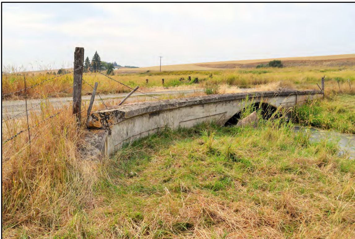
Figure A-110. Kelley Bridge (Field Number WCLB-16), east side; view to the northwest. Note the curved abutments and missing parapets.
